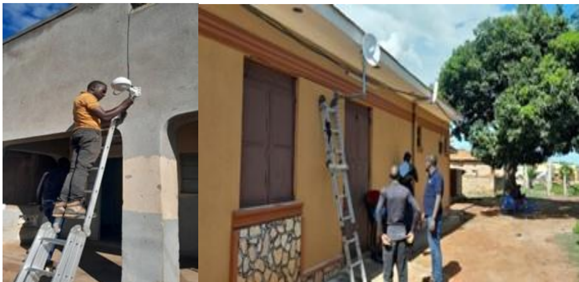
Caption: Network sites being installed at Atopi Market and the Kubere Information Centre, supported by APC and WACC.
